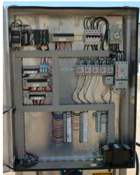
Control Center Components
