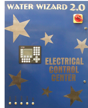
Electrical Control Center
