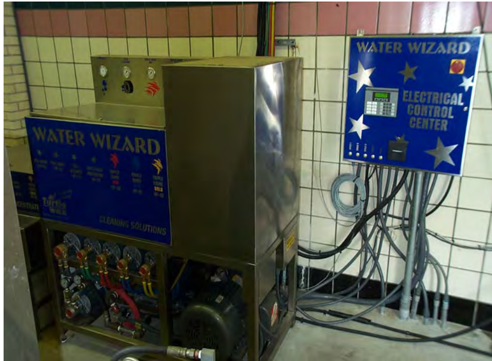
Pump Stand With Control Panel Removed
