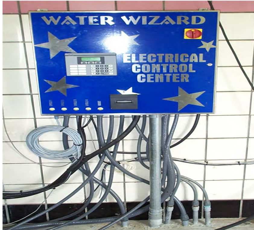
Control Panel Mounted to the Wall
