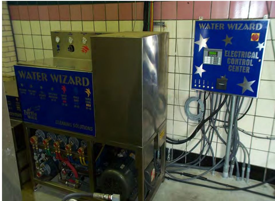
Pump Stand With Control Panel Removed
